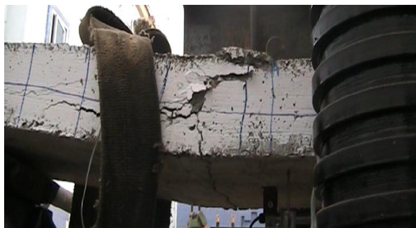
Fig. (7) Failure mode of slab S6-2O
