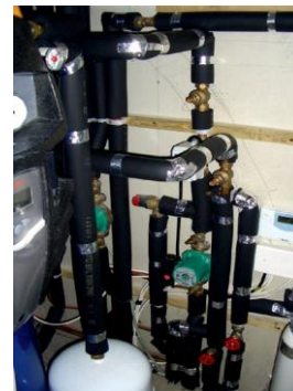
Fig. 34 A 'hot spot' was created in the airing cupboard by the MVHR unit and the pipework around the hot water cylinder. Additional insulation was later added to the pipework, which helped address the problem [9].
