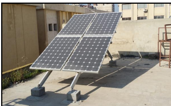
Fig.(1) : The photo of the solar cells modules.
