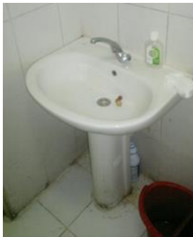
Fig. 8 Handwashing Sinks Source: researcher
