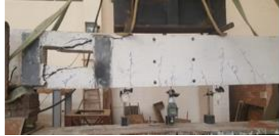
Fig. 8d Crack pattern for BSOC1
